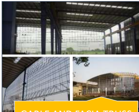
GABLE AND FACIA TRUSS WITH CABLE TRAY
